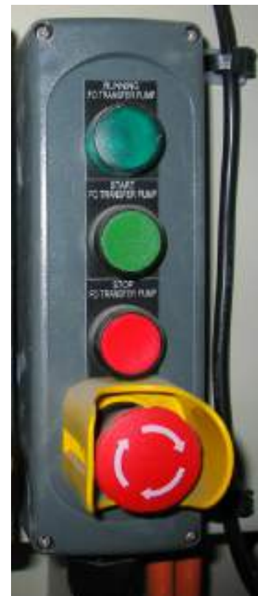
Figure 5-17 FO Transfer Pump Remote Control Panel
