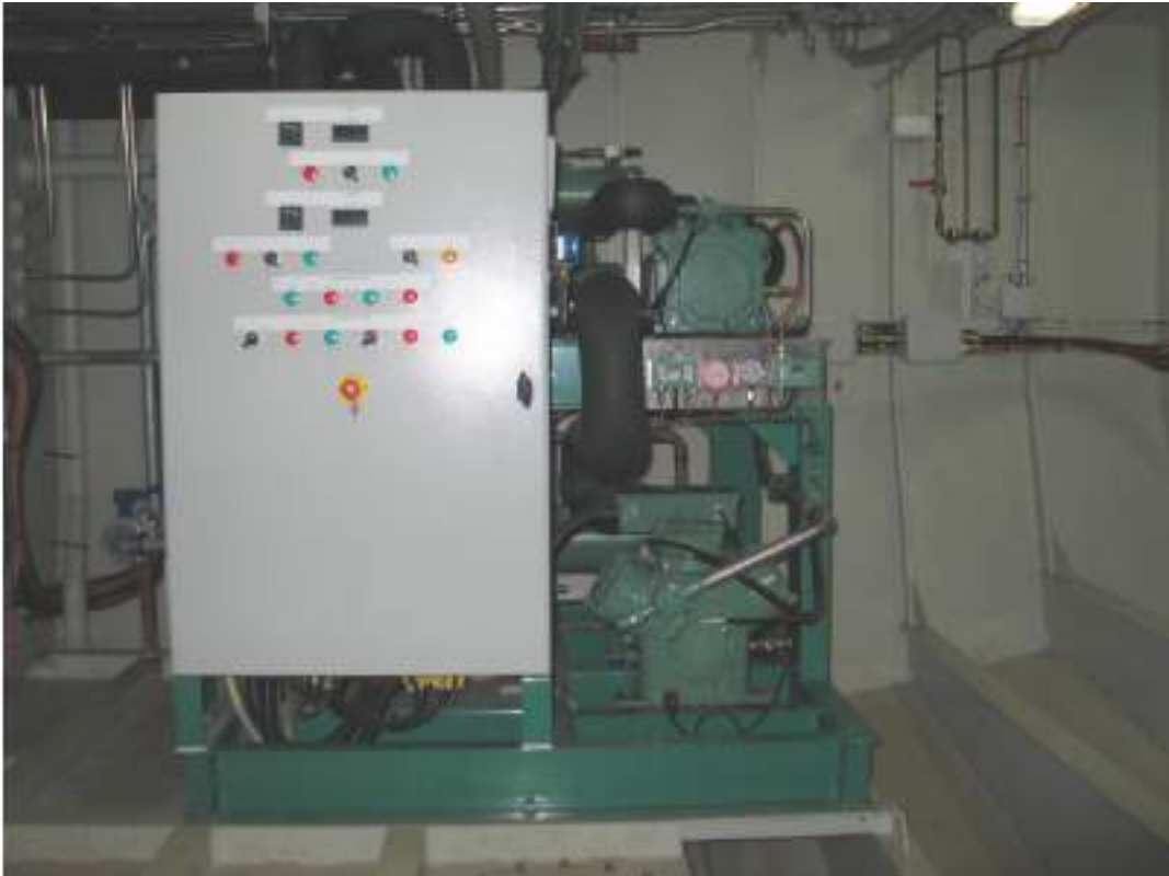
Figure 2-28 Storage_Room - Fish Hold refrigeration Plant
