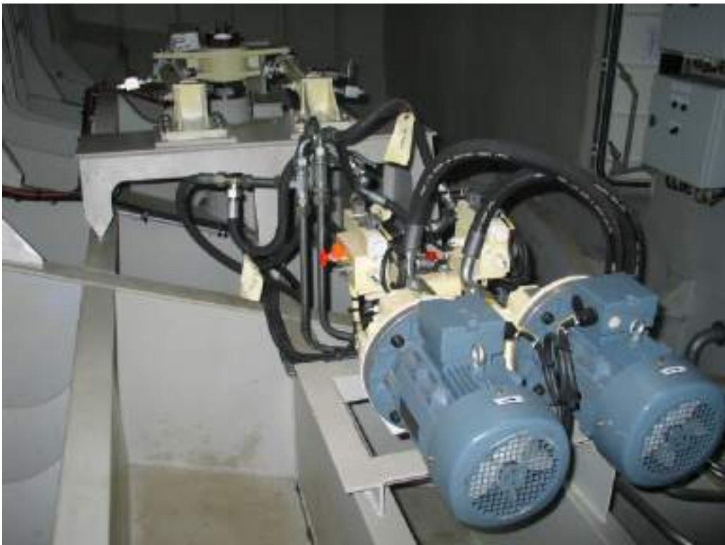
Figure 2-25 Steering Room - Hydraulic Power Unit Water Tank
