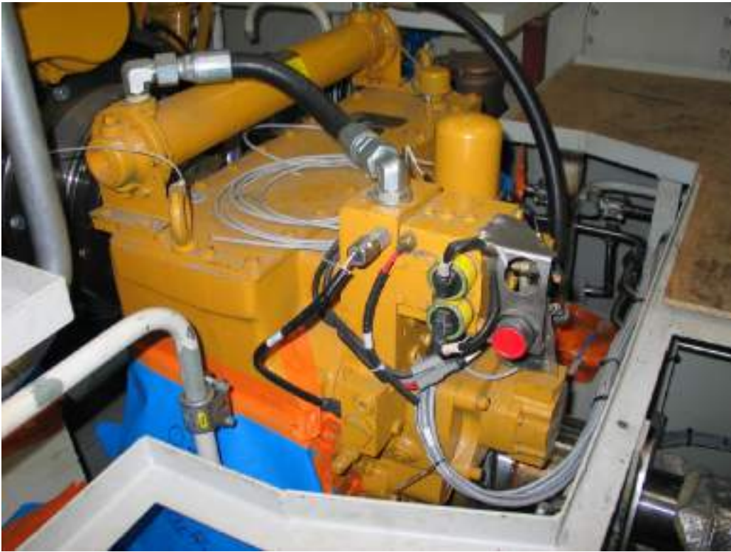
Figure 2-32 Engine Room - Gear Box
