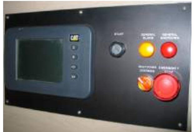
Figure 5-33 Engine Remote Control Panel
