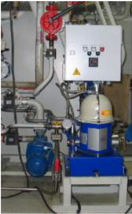
Figure 5-15 FO Transfer Pump and Separator Panel
