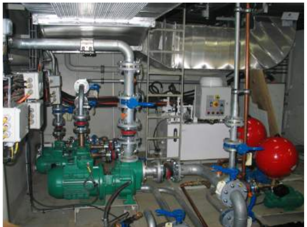
Figure 2-39 Engine Room - Stbd Side
