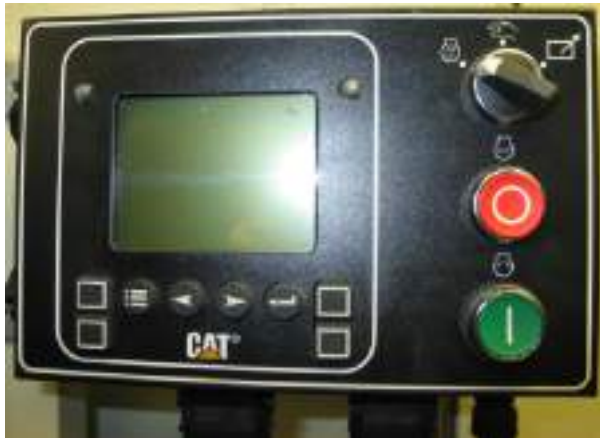
Figure 5-32 MECP-1 Engine Control Panel
