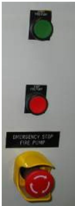
Figure 5-9 Main Switchboard - Fire Pump Control
