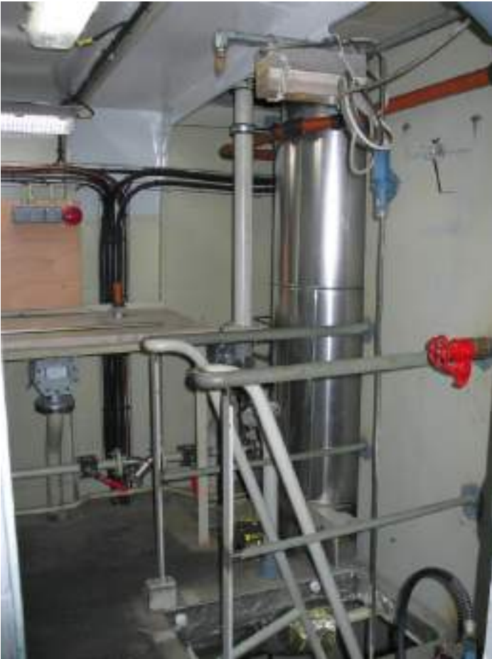
Figure 2-18 Workshop - Exhaust Silencer and Engine Room Ladder
