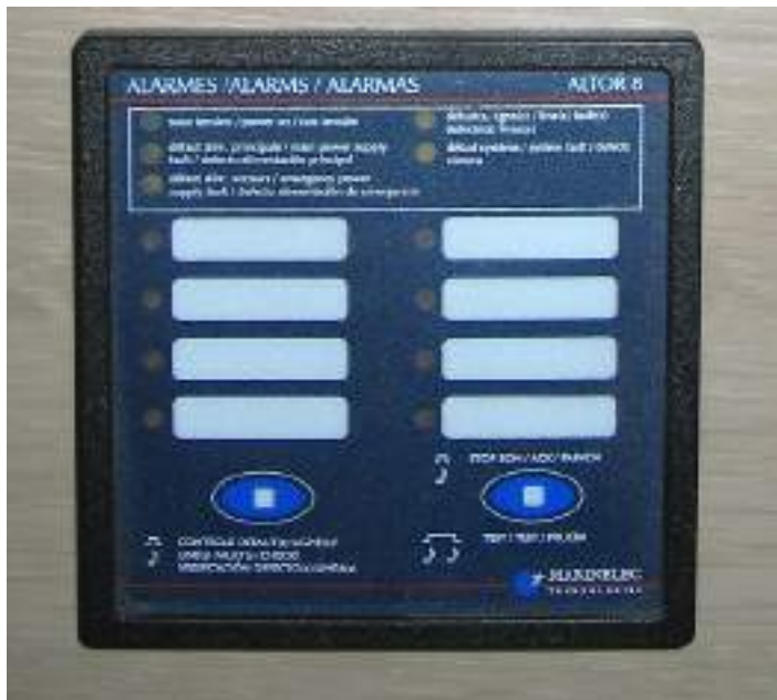
Figure 5-28 Bilge Alarm Panel
