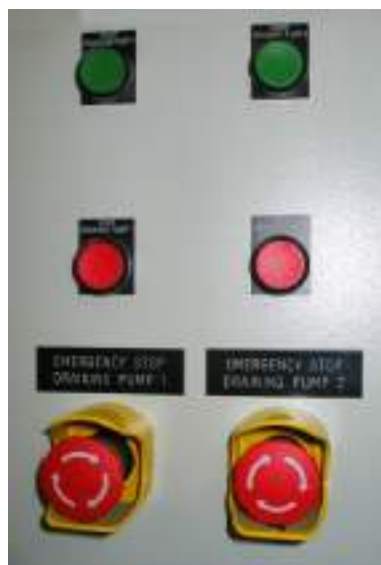
Figure 5-13 Main Switchboard - Bilge Pumps Control
