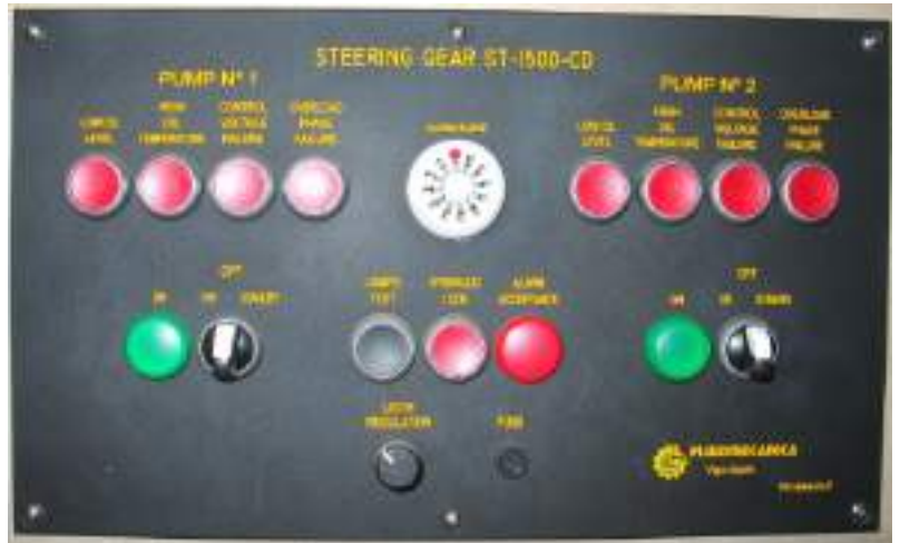
Fig5-2 Bridge Remote Control Monitoring and Alarm Panel
