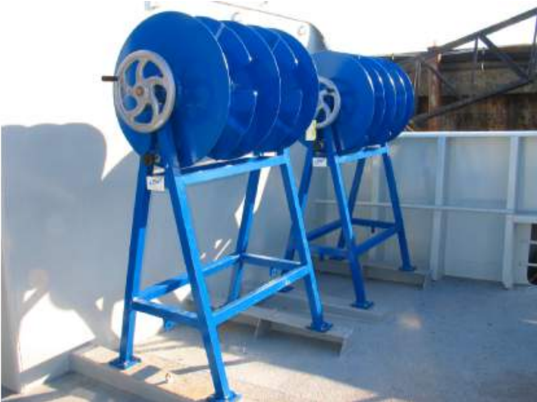
Figure 2-5 Stbd Aft Deck – Manual Line Drum
