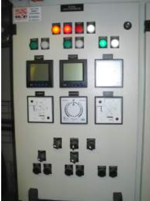
Figure 5-23 Main Electrical Switchboard - Production Cell
