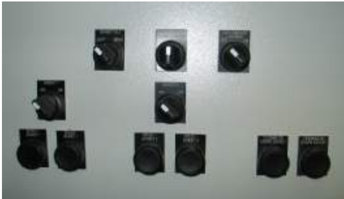
Figure 5-24 Main Electrical Switchboard - Production Cell
