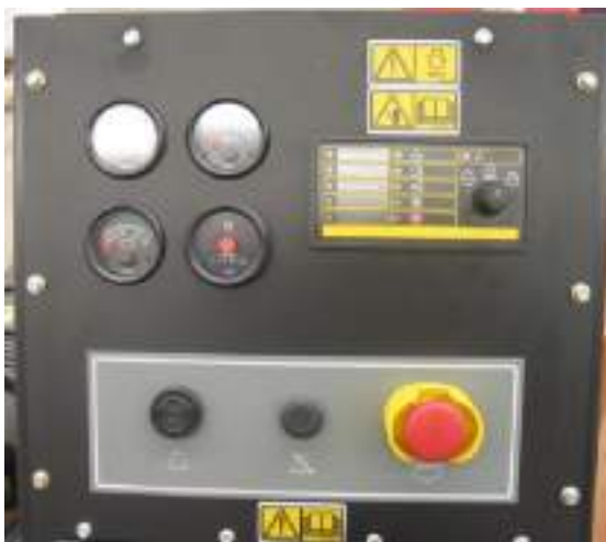
Figure 5-26 Genset Control Panel
