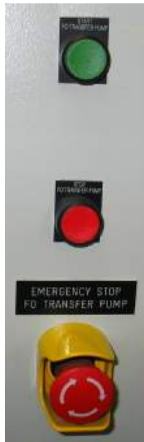
Figure 5-16 Main Switchboard - FO Transfer Pump Control
