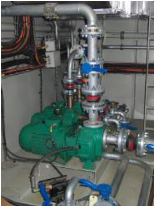
Figure 5-37 SW Cooling Pumps
