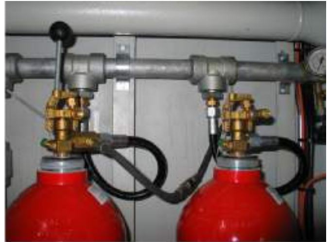
Figure 5-21 Mechanical Release Lever (Cylinder 1) and Pneumatic Release (Cylinder 2)
