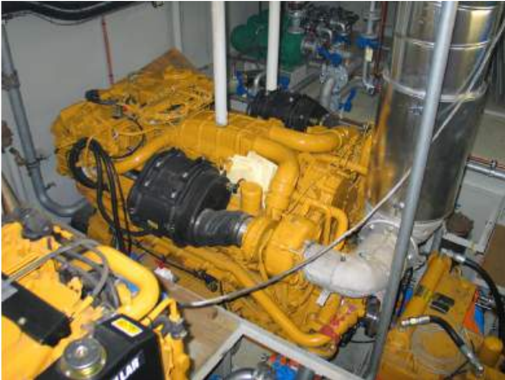
Figure 2-30 Engine Room - Main Engine
