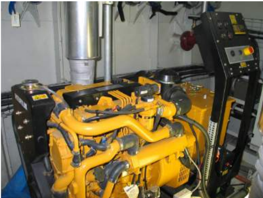
Figure 2-33 Engine Room - Port Generator
