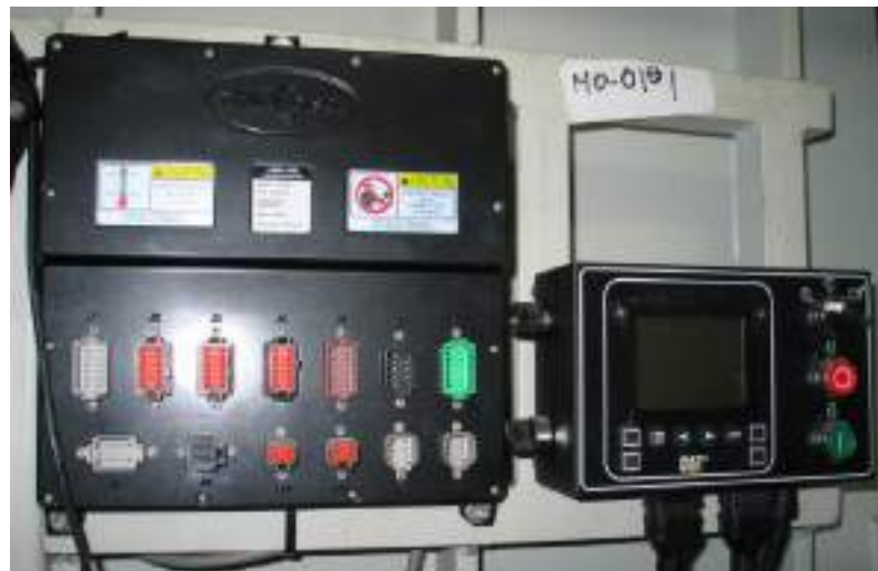
Figure 5-35 EC300 Controller & MECP-1 Eng. Control Panel
