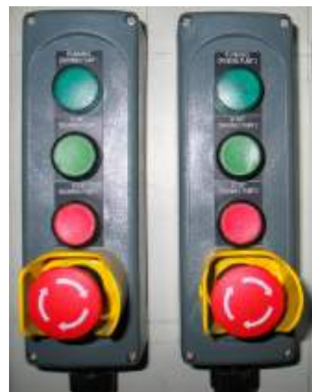
Figure 5-14 Bilge Pumps Remote Control Panels
