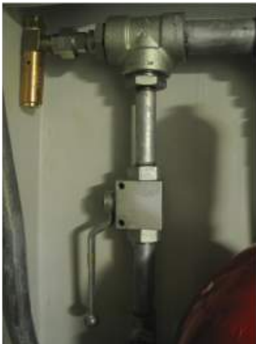
Figure 5-22 CO2 Isolating Valve
