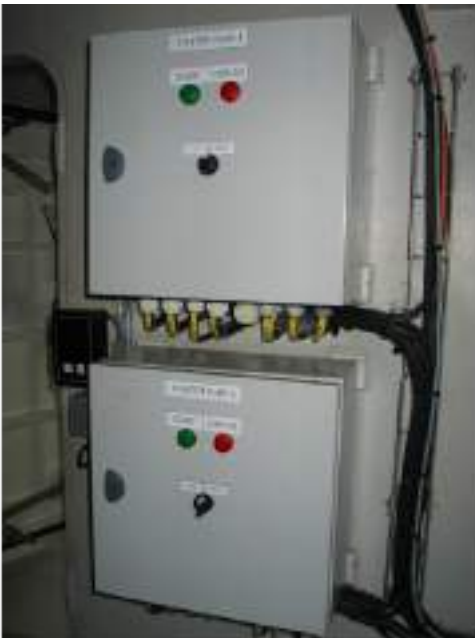
Fig5-1 Steering Gear - Electrical Starters HPU1 & 2
