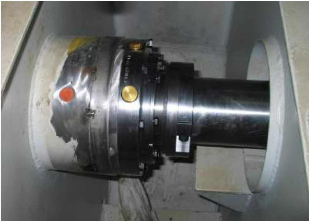
Figure 2-29 Storage Room - Stern Tube
