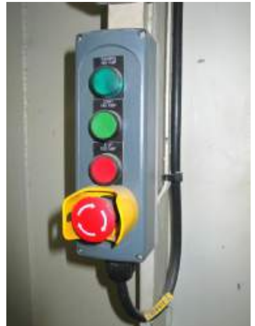
Figure 5-10_Fire Pump Remote Control
