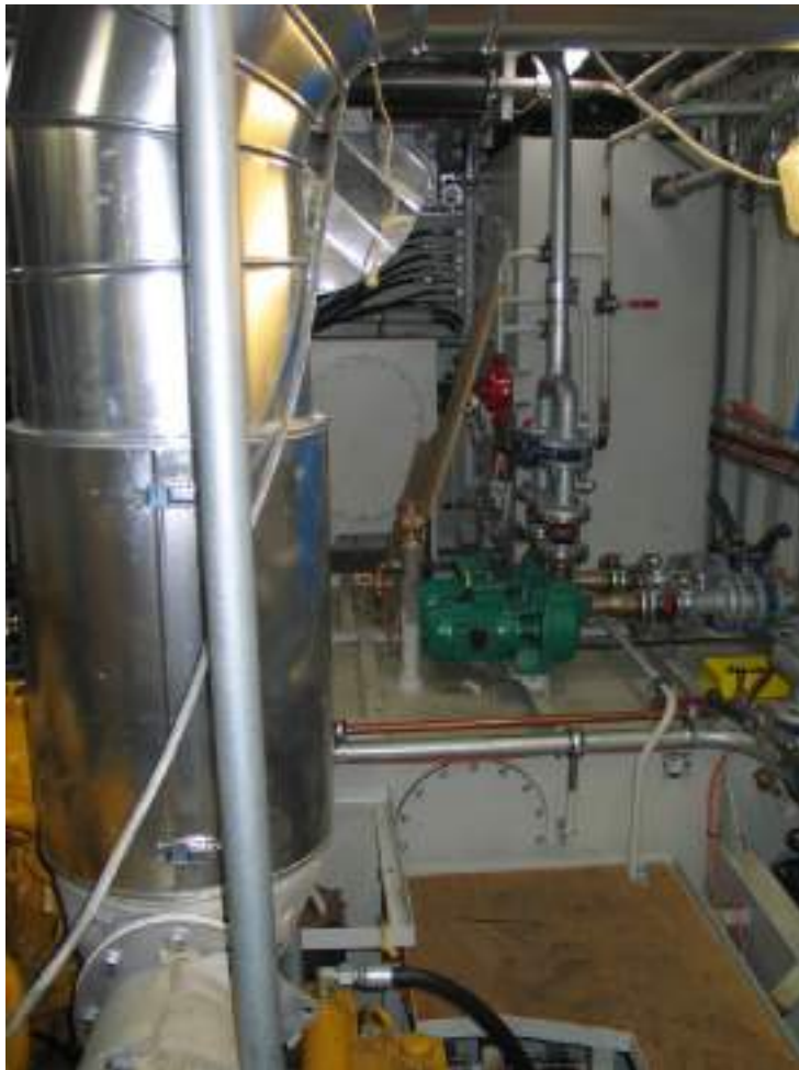
Figure 2-38 Engine Room - Stbd Side
